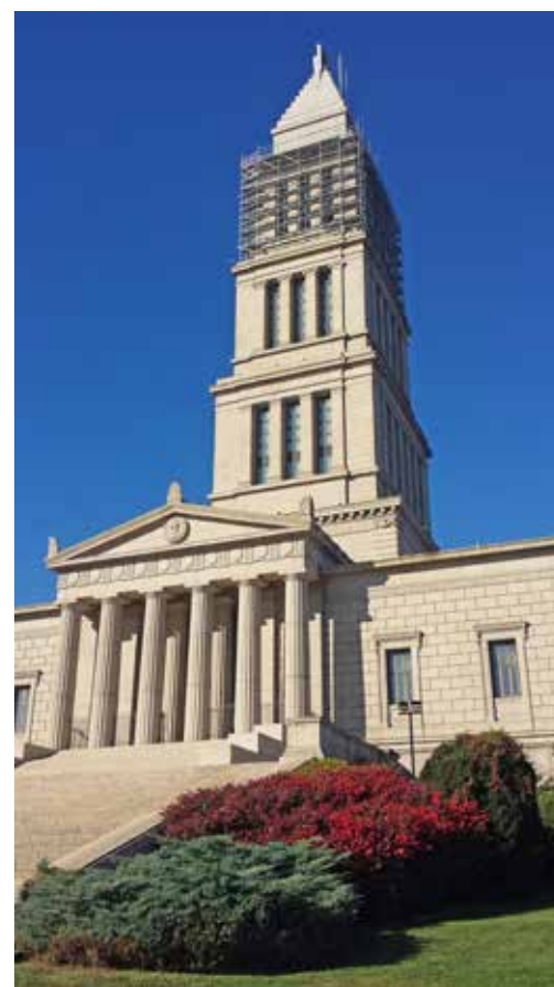
The scaffolding on the upper tower used by operative Masons to re-grout the granite blocks.
